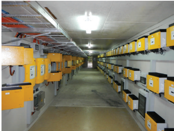
Figure 5: PV inverter and battery Inverters for a hybrid system (Source: Simon Troman)
