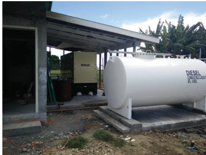
Figure 6: Fuelled generator installed in a hybrid system (Source: Clay Energy)
