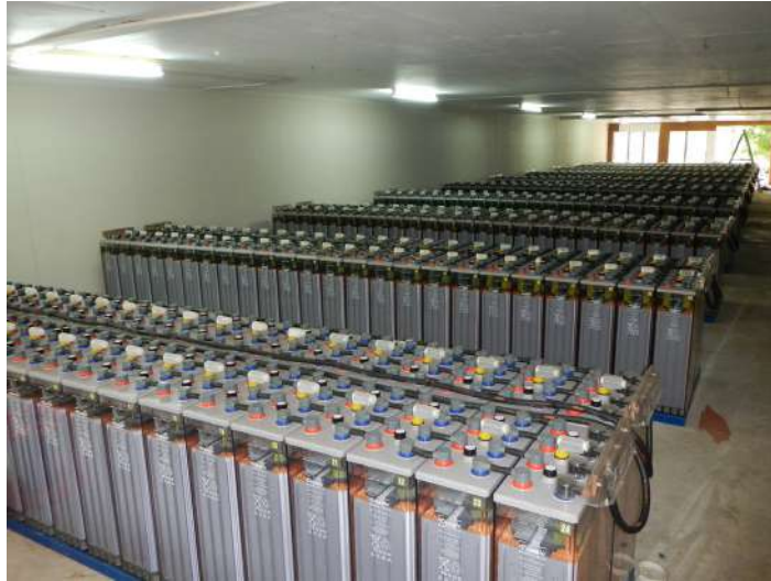
Figure 4: Battery bank for a hybrid system (Source: Simon Troman)
