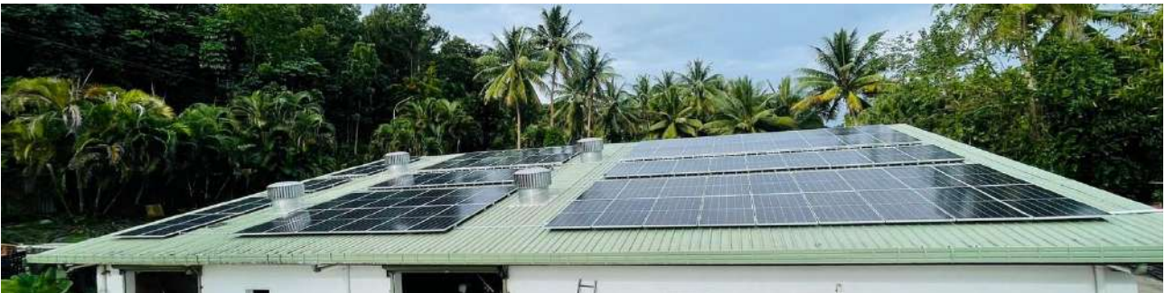
88kW PV system-Warwick-Hotel
