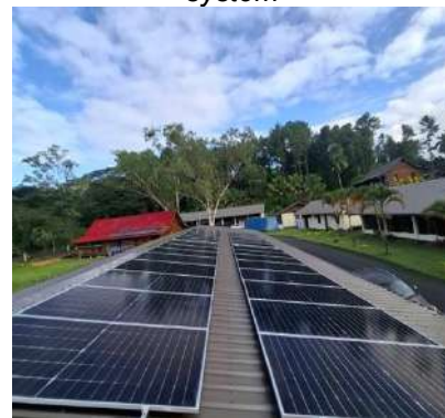
CATD 20 kW system
