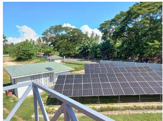
Systems installed by SEI API Member: Superfly Limited- Solomon Islands
