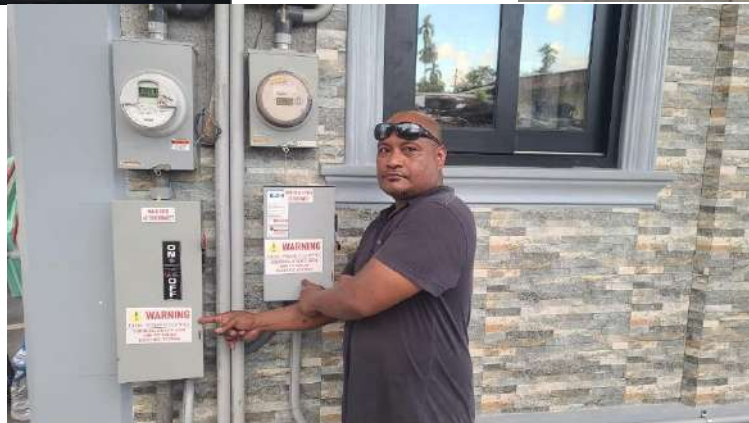
15kW PV System and 10kWh Battery system on grid
