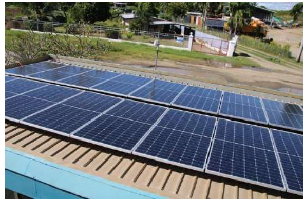
30kW PV system at Bluegas Vuda
