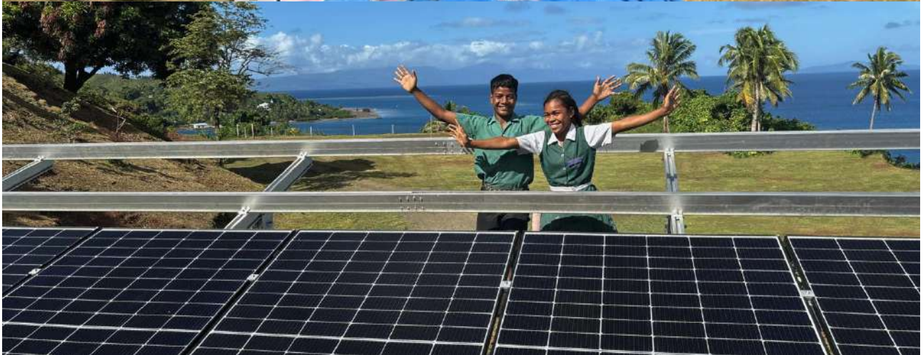
Solar Systems for Schools in Fiji - Installed by SEI-API Member Its Time Foundation
