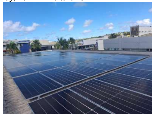
Palas Auto 40kW P array with 60kWh battery system
