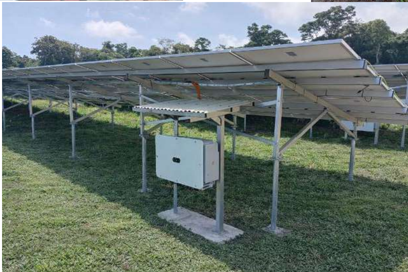
3MWp Solar Farm Vanuatu Systems installed by SEI-API member Pacific Engineering Projects Fiji
