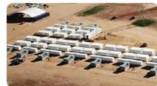
Battery Energy Storage System (BESS)
