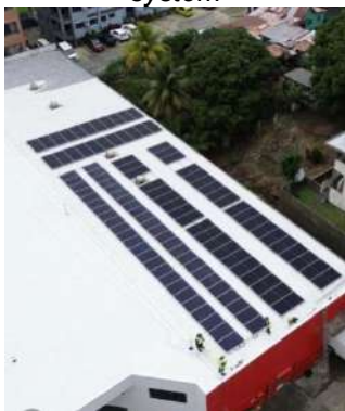
Roopesh Gift Shop 38 kW PV array with 60kWh battery
