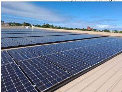
Narhari HQ 50kW PV array with 100kWh battery system
