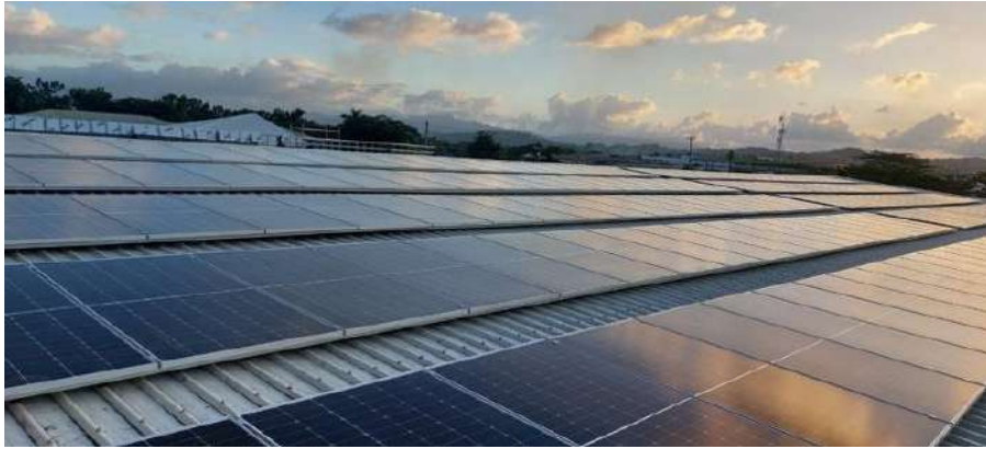
150kW PV system at Extra Labasa
