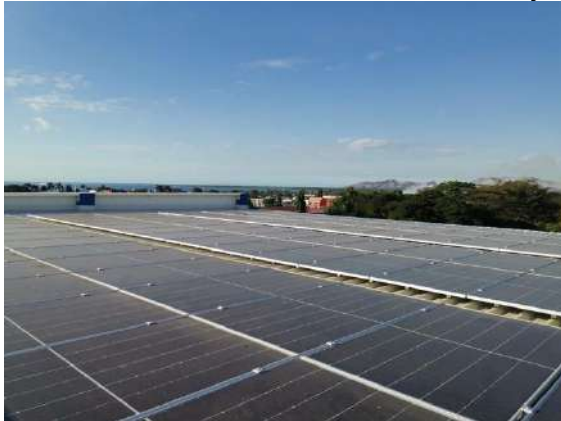
80kW PV system at Lautoka Police Station
