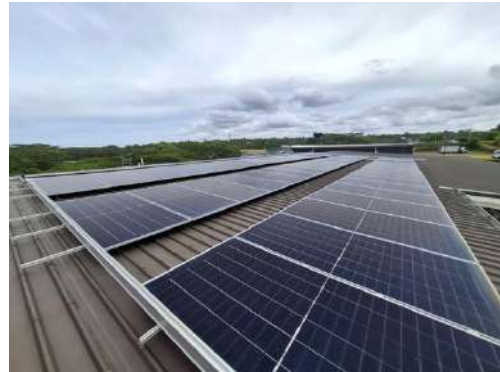
Grace Road 60kW system
