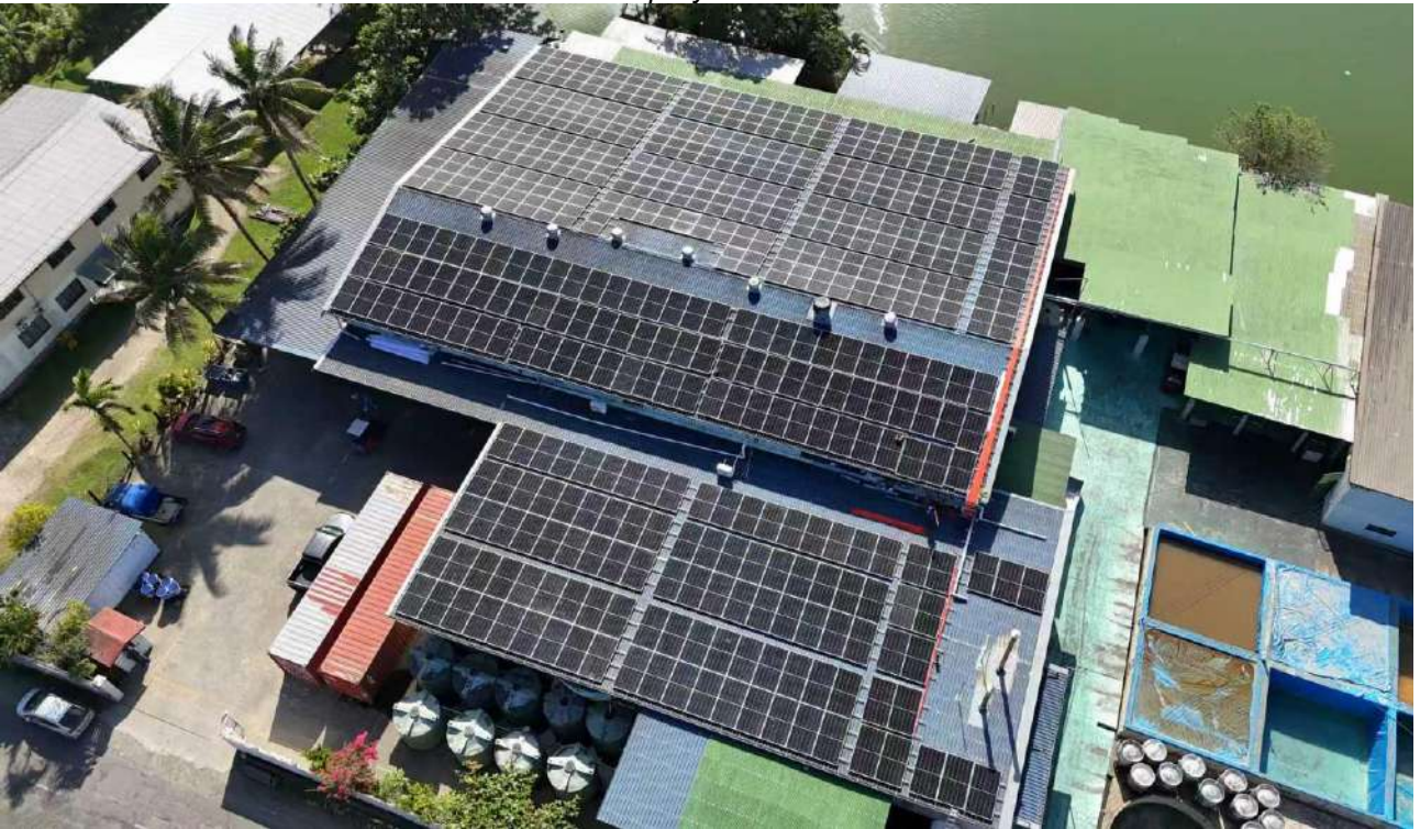
310 kWp system Vanua
