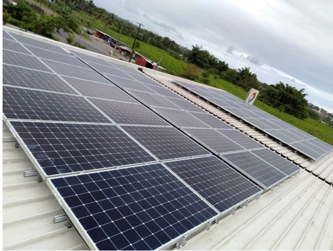
Figure 6: Array on House Roof
