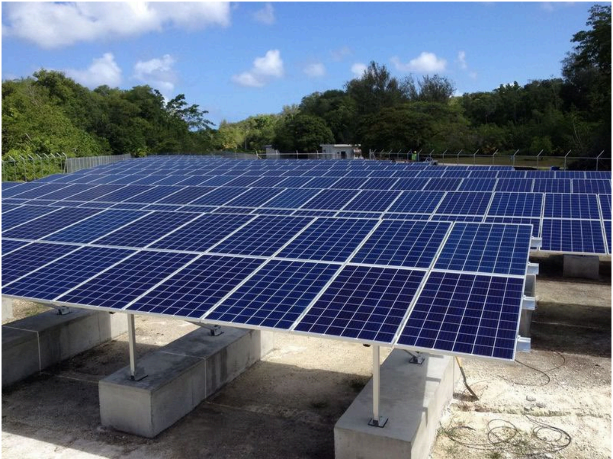
Figure 3: Ground Mounted Solar Array
