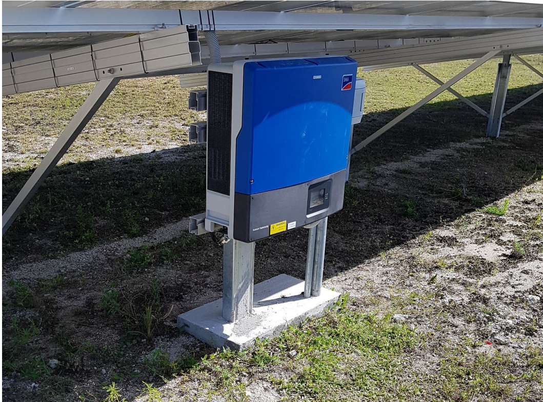
Figure 4: Showing Inverter and Frame
