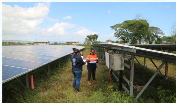
Solomon Power Staff inspecting one of their systems
